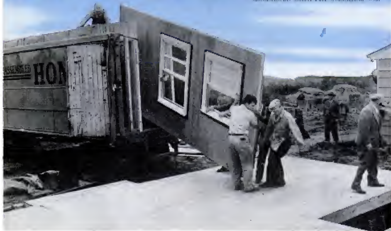
This is the way a completed wall section of prefabricated home is unloaded onto the slab foundation Harsco-Baker Corp., Port Washington, Wis.
